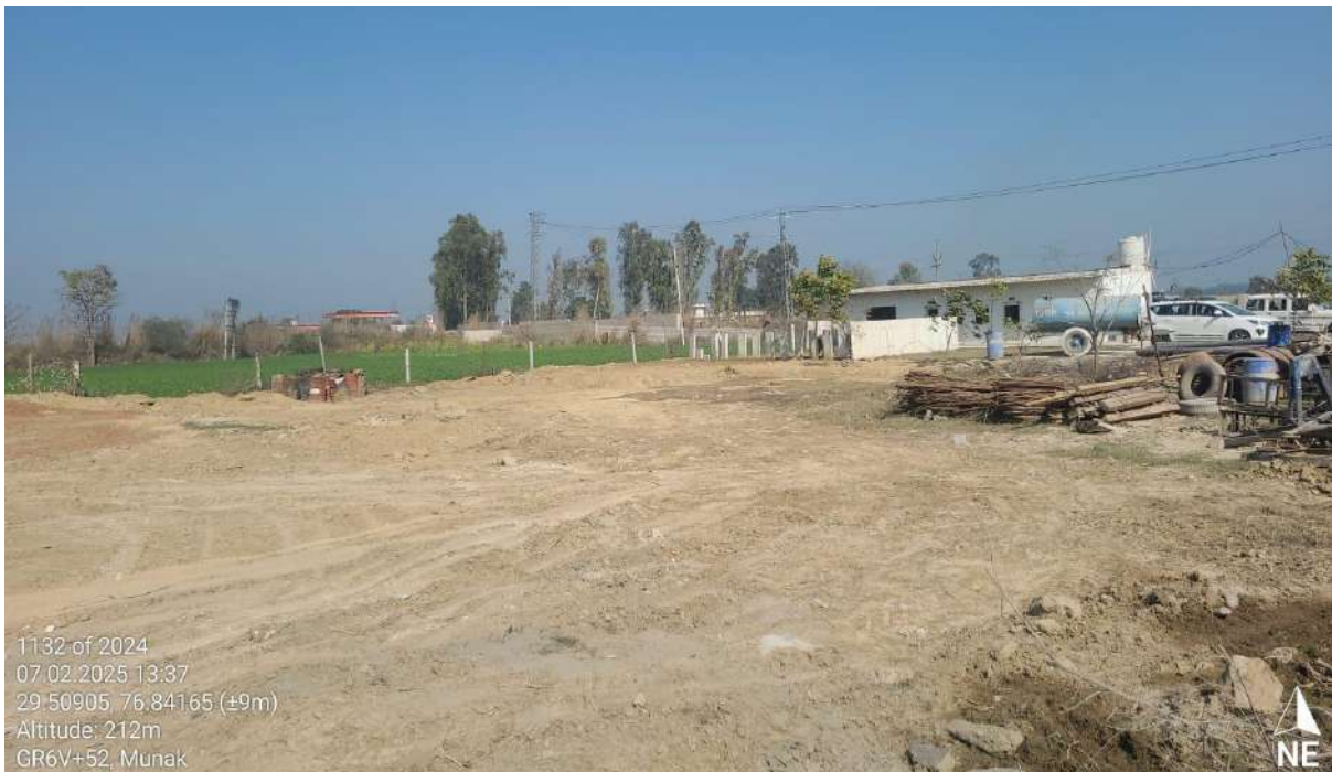
Photograph 6: Inadequate arrangements for dust suppression within the premises.
