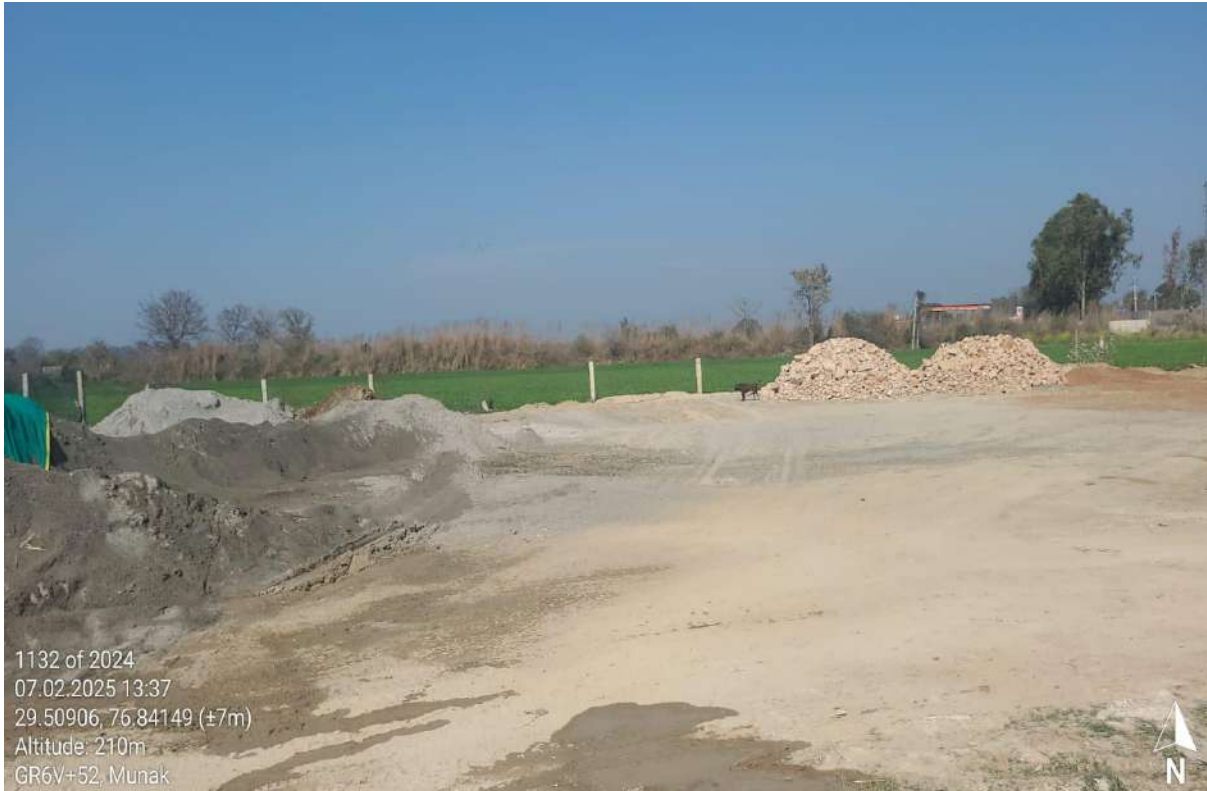
Photograph 5: No boundary wall, green belt and wind breaking wall provided.
