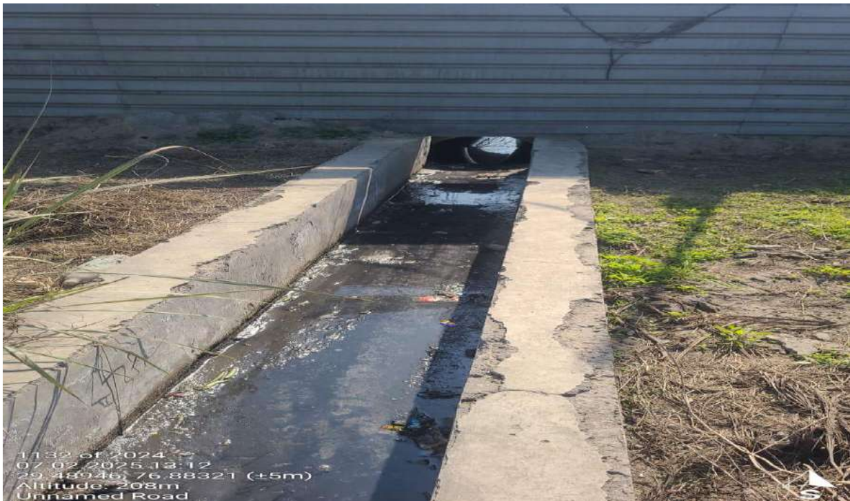
Photograph 2: Arrangement made to bypass STP and discharge untreated sewage into the nearby drain.
